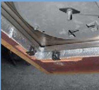
Asbesttextil in Kochherd
